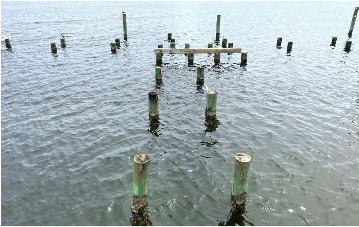
View of remaining piles from the damaged dock (looking south)
